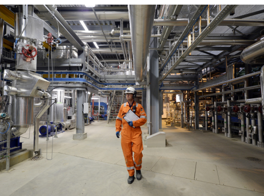
Lincolshire incinerator. United Kingdom.
